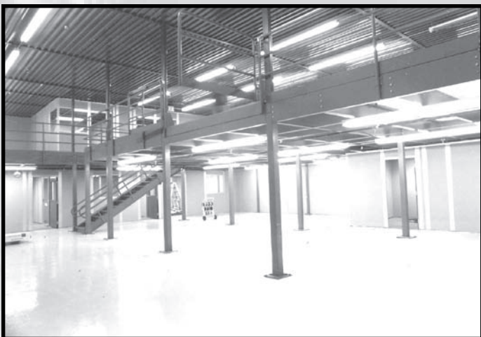
Mezzanine structure optimizes the use of available floor space permitting the installation of offices and laborato-
