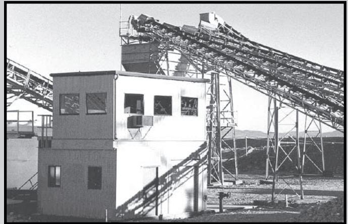
Personnel and equipment within the control rooms are isolated from high temperatures, dirt and noise. The building is self-contained, complete with emergency power systems, housing the computerized operating system at this automated cement batch plant.
