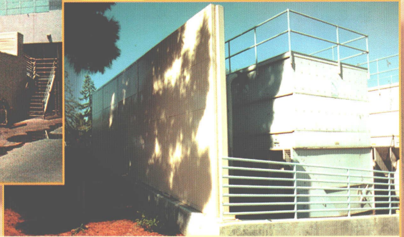
Soundwalls reduce community cooling tower noise.
